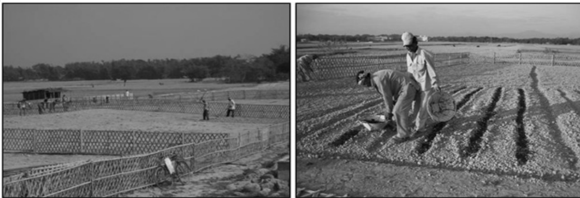
Fig. 6 Properly stored and maintained top soil with mulch treatment around a drilling site in Assam, Northeast India
