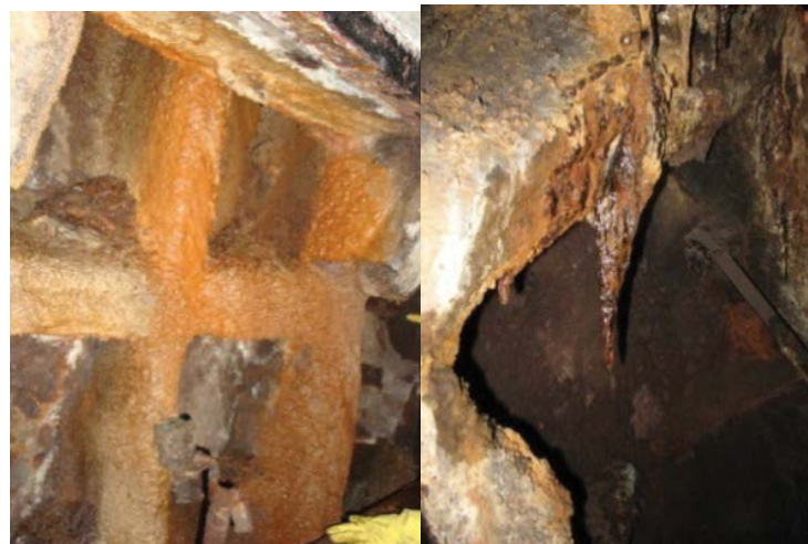
Fig. 4 Growth and leaching with a rusty wet coating (a); Stalactite on the lining stiffener rig (b).
